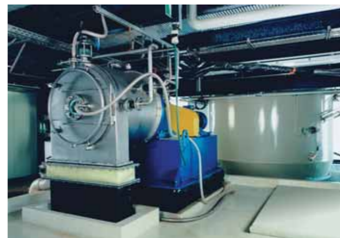
Details from a pickling bath liquor regeneration unit
