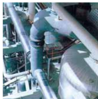
Vacuum evaporators for brine concentration
