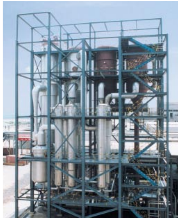
3-effect falling film forced circulation evaporation plant heated by thermal vapour recompressor for waste water from sodium glutamate production. Evaporation rate: 50 t/hr
