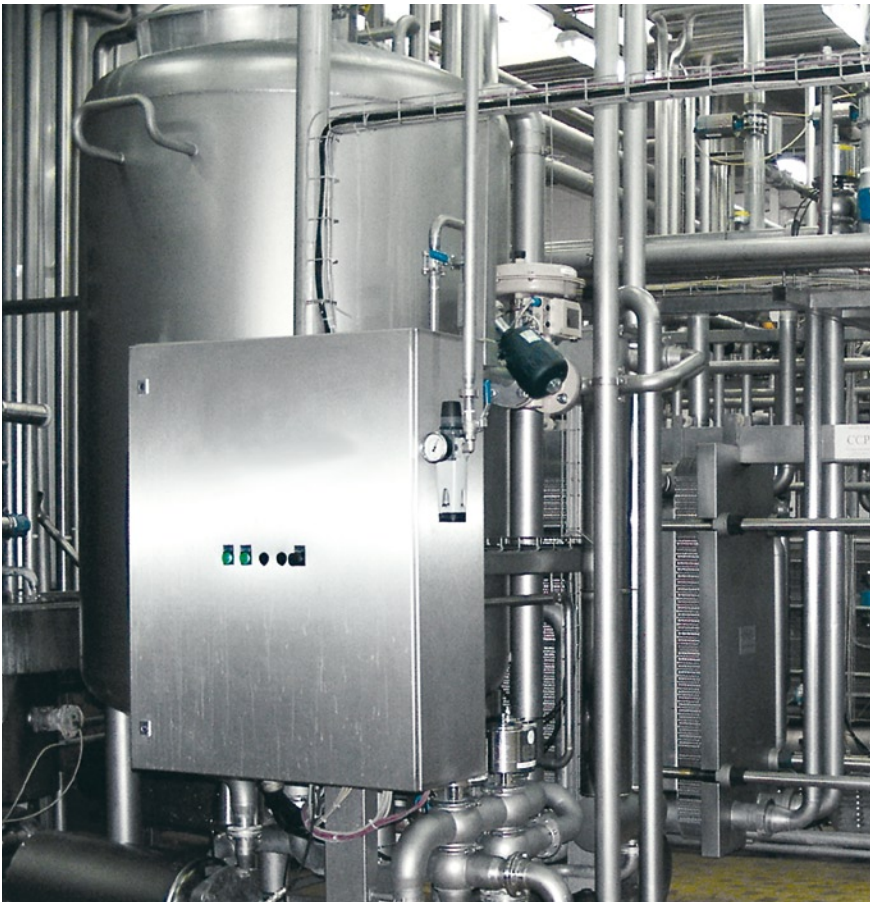
Stratified storage tank
